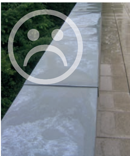
Zinc hydroxide formation due to insufficient slope
